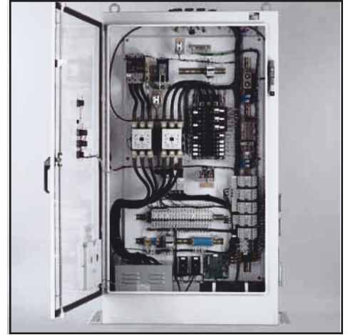
Power Distribution, Interior: 78" x 48" x 18"
